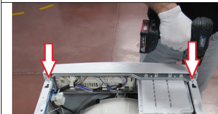
3.11.1 Tighten two screws fixing control panel.
